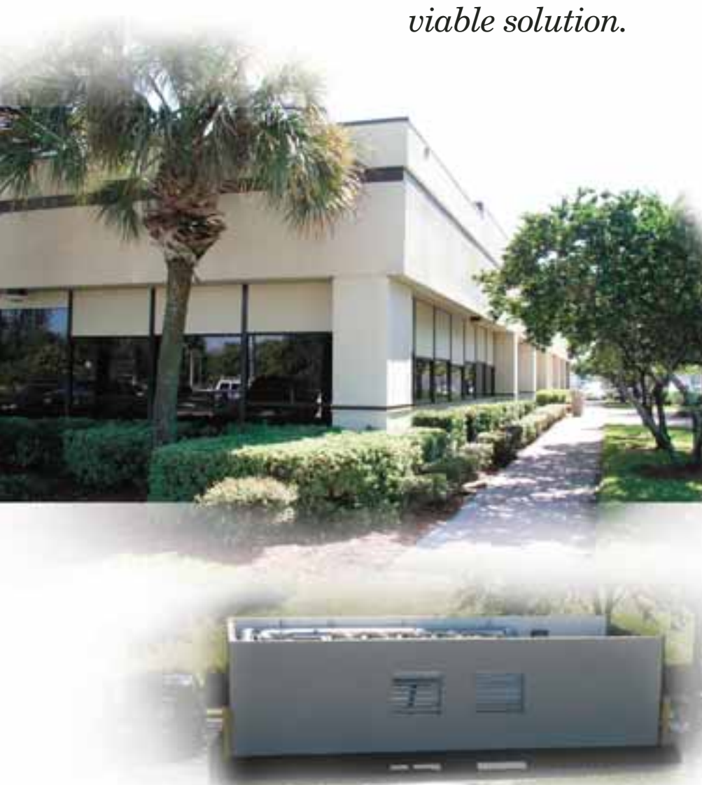
The air-cooled chiller was located in a compact, existing enclosure near the rear of the building.
