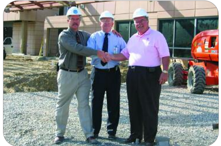
Mike Gardner (center) of LRMC with Rick Gerun and Jim Sparling of Trane.
